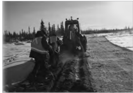
For these sections of the route, the cable is installed directly in a trench, in the active layer of the permafrost
