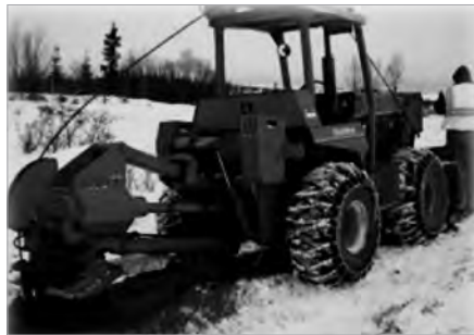
This section can be installed during the summer/fall seasons using a traditional cable plough.
