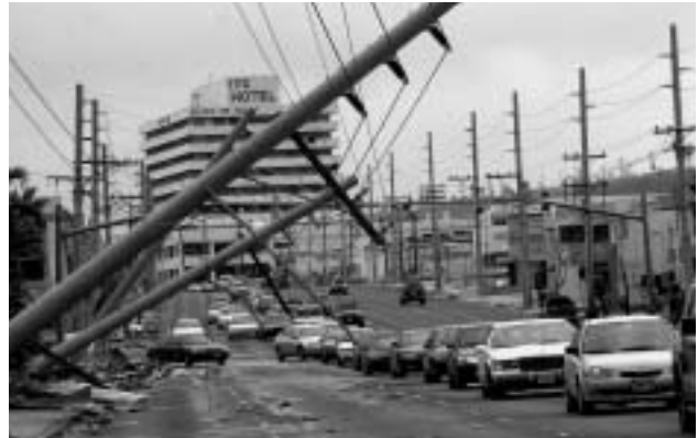
Power poles along Marine Drive in Tamuning were tilted midway as a result of Super typhoon Pongsona in December, one of two storms that blasted Guam in 2002. Photo: Pacific Daily News
